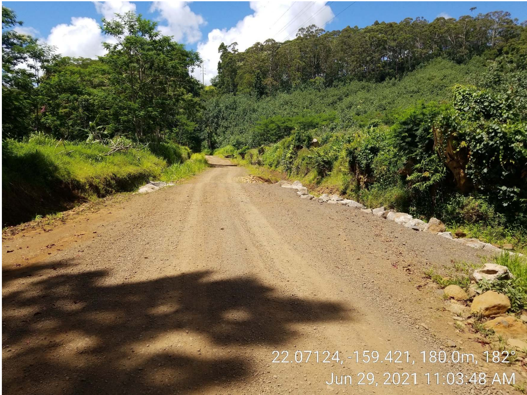
Figure 12: Photograph of the (crudely repaired) passible road at the New Crossing
