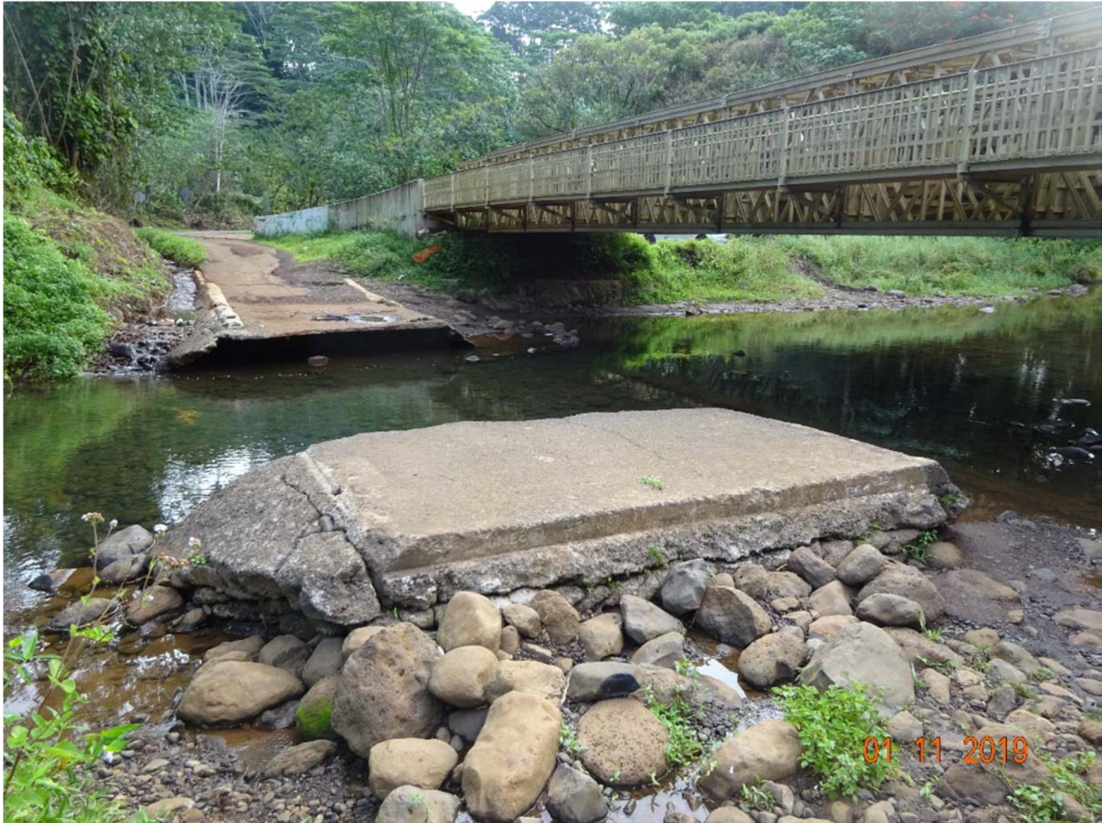
Figure 8: Photograph of the Keāhua Stream Ford post-flood, view to East (adapted from Hart Crowser, Inc. 2019)
